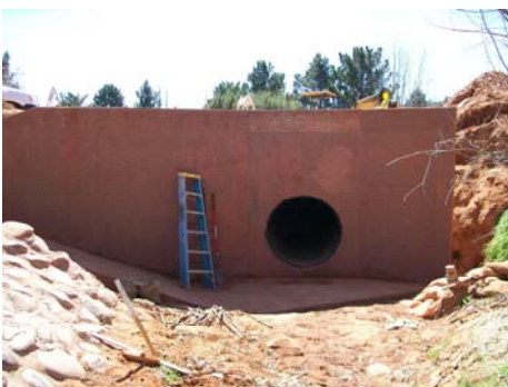
The District designs and constructs storm drain systems such as the system in the Village of Oak Creek shown above when there is space and required right-of-way available or attainable. Similar projects have been completed in areas such as Lake Montezuma and Black Canyon City.
