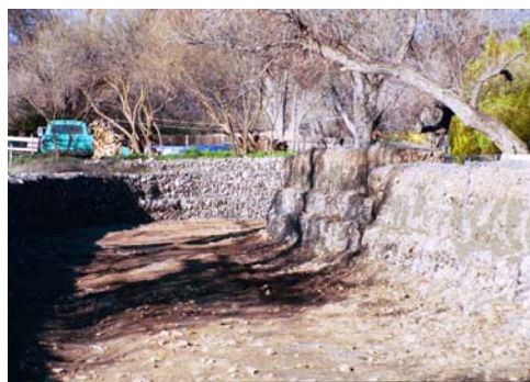
Lee Wash in Lake Montezuma was lined with gabion baskets on the sides and gabion mattresses on the bottom. A similar project, in its preliminary stages, is being considered along South Rocky Boy Wash in Peoples Valley to prevent continued erosion into the properties platted along the wash in the early 1970s.
